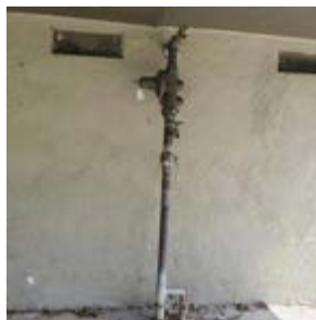
Common Water Main
